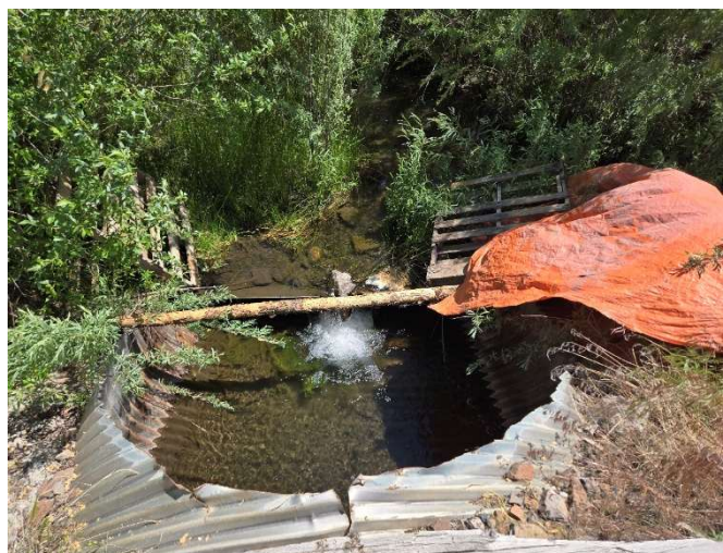
Fig 35. TU. View of the displaced culverts on Maggie Creek, upstream. A diversion (wood and orange tarp) was built to help control water during high flow periods (June 2025).
