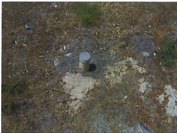
Suspected septic system clean out on south side of Senior Center building
