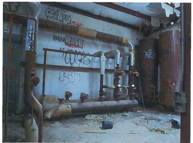
Boiler Room piping and water tanks
