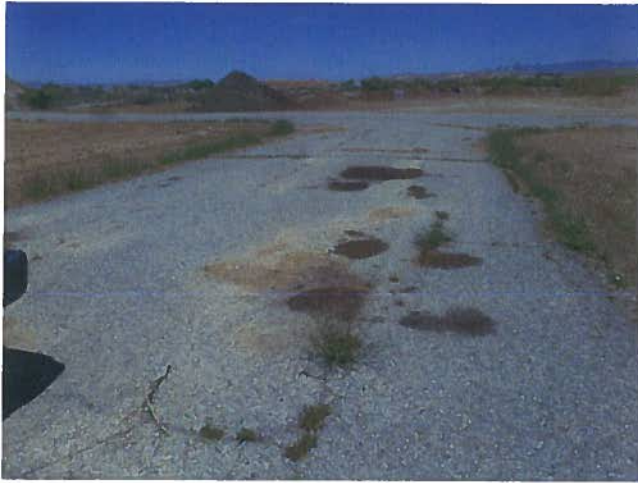
On-site pavement staining, north of small greenhouse
