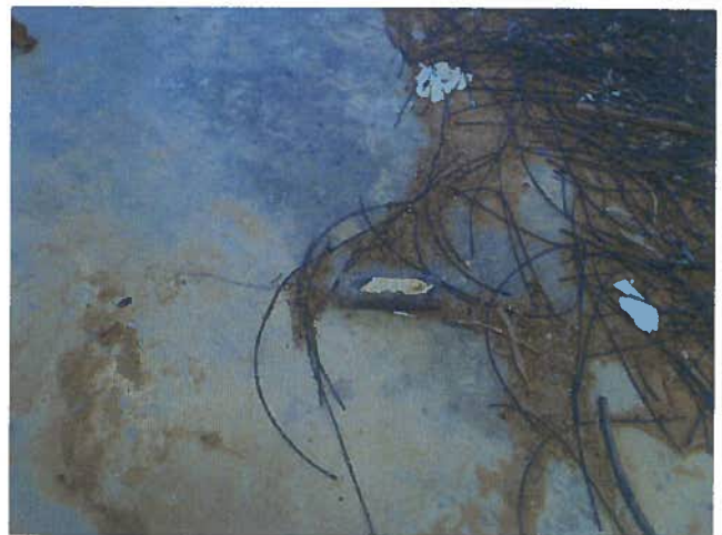
Fluorescent light ballast on floor
