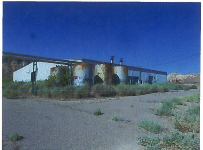
On-site ASTs, northeast corner of Packing Plant
