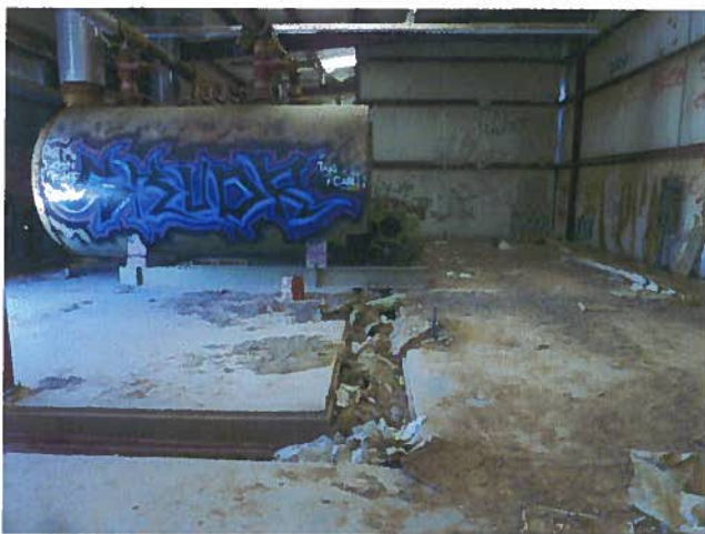
Packing Plant Boiler Room fuel tank
