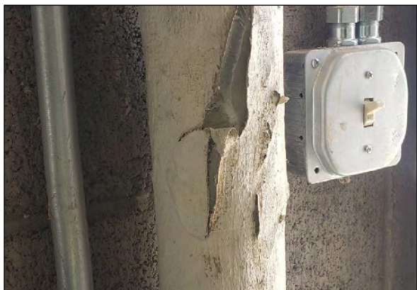
Identified damaged friable ACBMs (pipe insulation)
