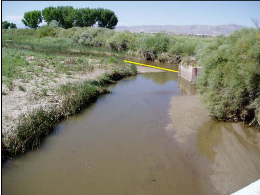
Site: Walker River Site # WR6 – Miller Lane Bridge (B-1519) (Photo taken from bridge, looking upstream)
