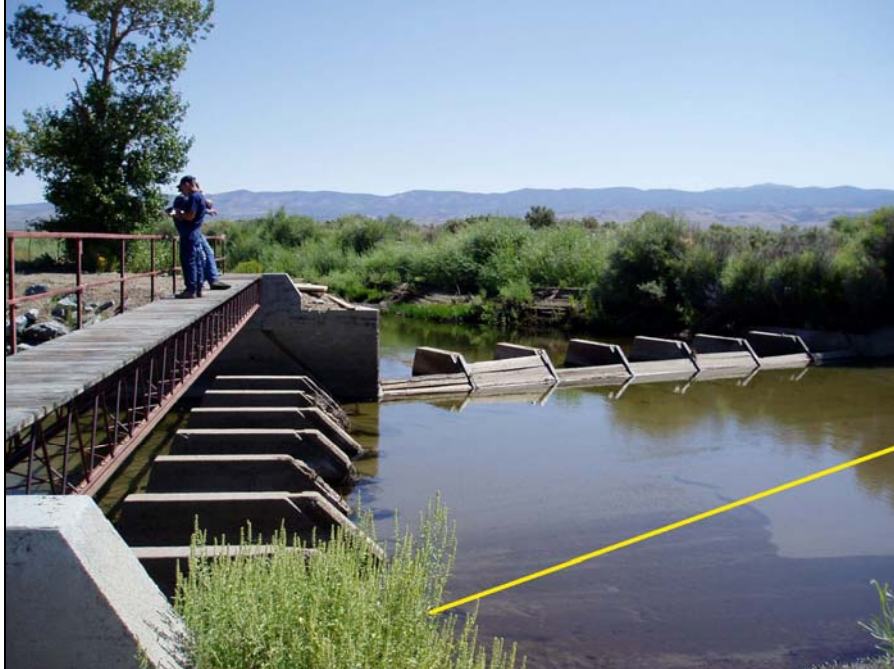
Site: West Walker River Site # WW10 – Summers Ranch (Topaz Diversion) (Photo taken from west bank, looking downstream)
