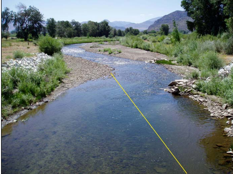
Site: West Walker River Site # WW8 – Cunningham Lane Bridge (B47C-12) (Photo taken from bridge, looking upstream)
