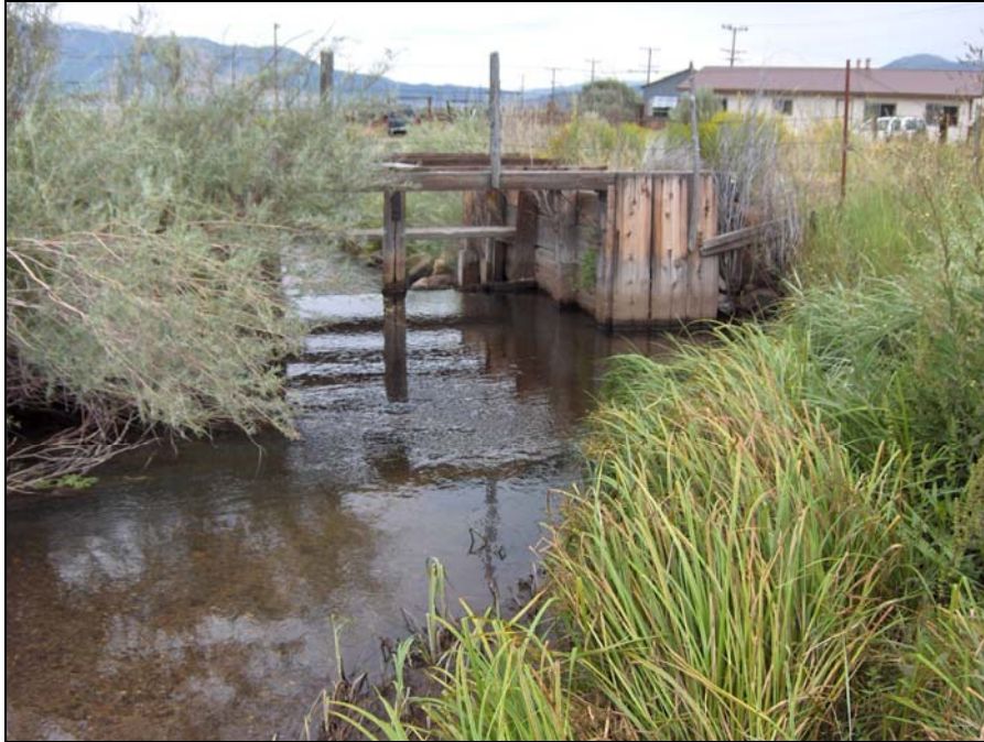
Site: East Walker River Site # EW5 – Point Ranch (Photo taken looking downstream towards diversion)
