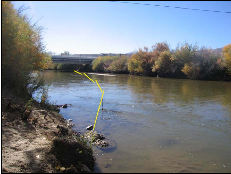
Site: Walker River Site # WR3 – Bridge Street (Yerington) Bridge B-1408 (Photo taken from east bank, looking upstream at bridge)
