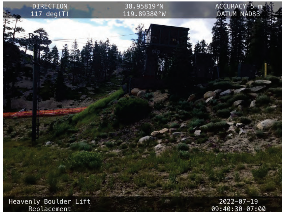
Photo 2. Existing Boulder Lift upper terminal to be replaced in existing location. A temporary access route will be constructed on down slope side during construction. No impacts to regulated waters from replacement of the upper terminal.
