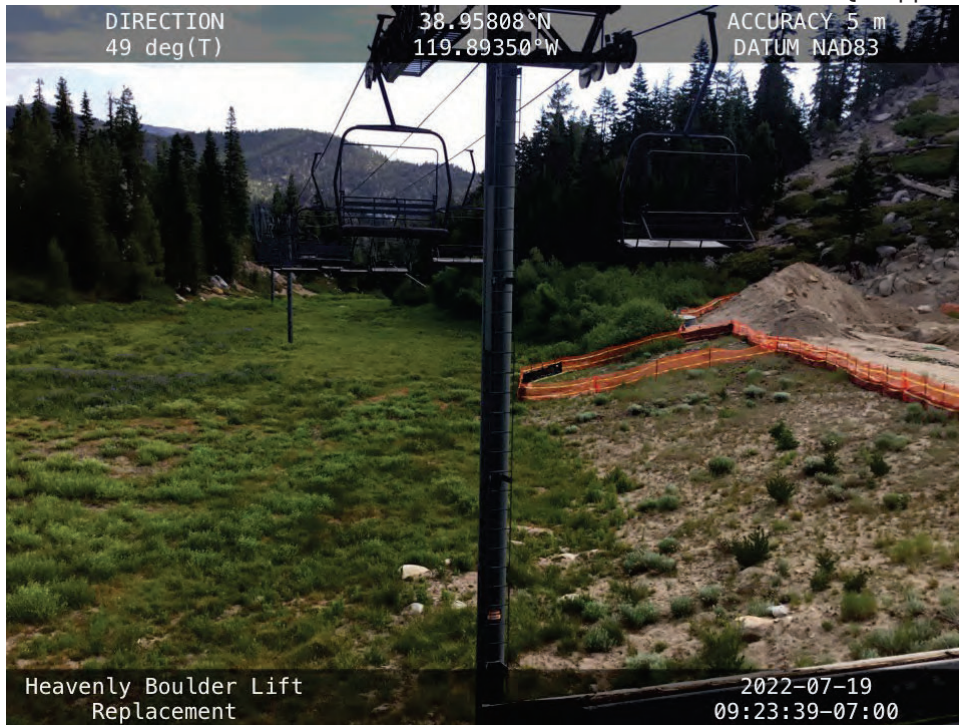
Photo 3. Existing lift tower within wetland to be removed (shown in background). Tower will be cut at base and flown from site. Location of proposed new tower 10 will be located within a similar location creating 741 sf of temporary impact during construction, to be restored, and 225 sf of permanent wetland from location of the tower footing (15' x 15'). A temporary access route utilizing construction mats will be located under lift alignment and will be restored upon project completion.
