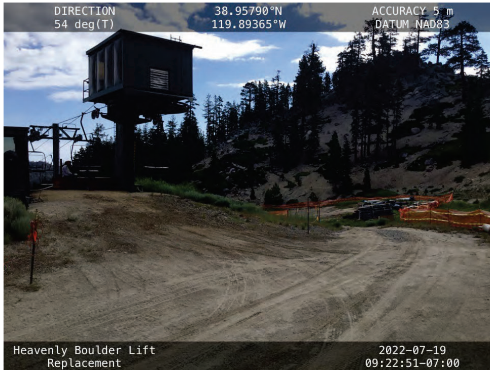
Photo 1. The existing Boulder Lift upper terminal to be replaced in its existing location. Entire terminal is located in uplands and access to site will be through existing summer access road.
