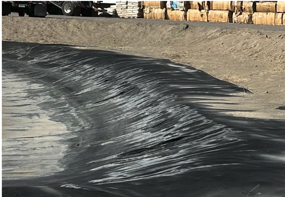
Photo 3 – Stormwater pond pre-construction primary liner north sidewall degradation 11/11/24.
