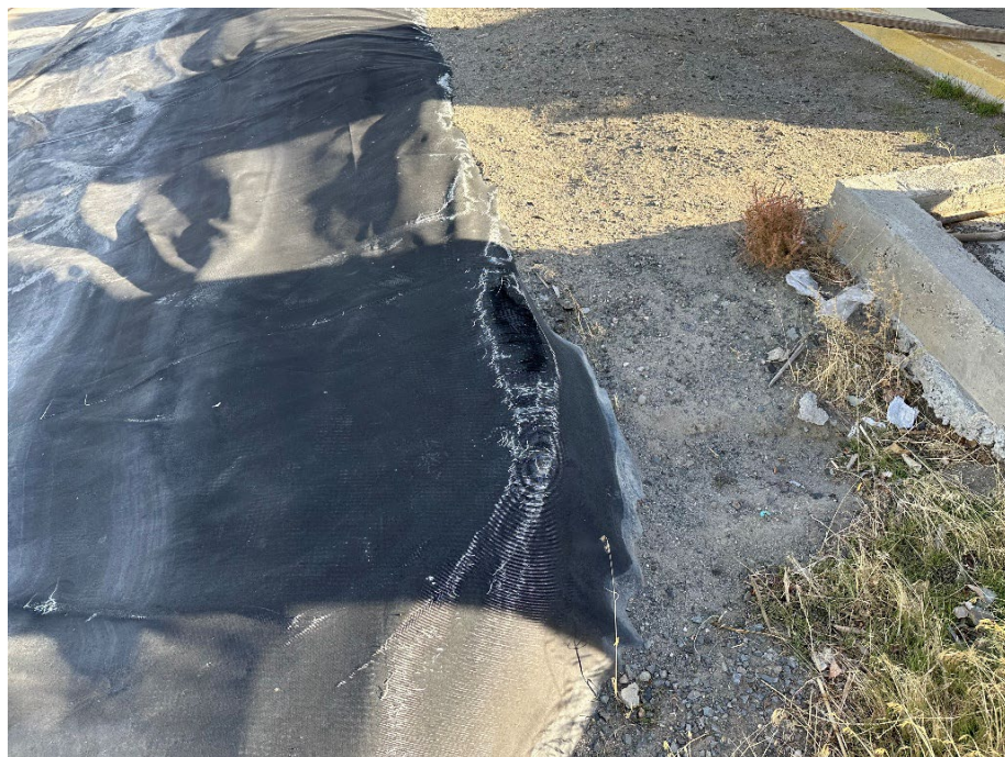
Photo 6 – Stormwater pond pre-construction top of liner tear 11/11/24.
