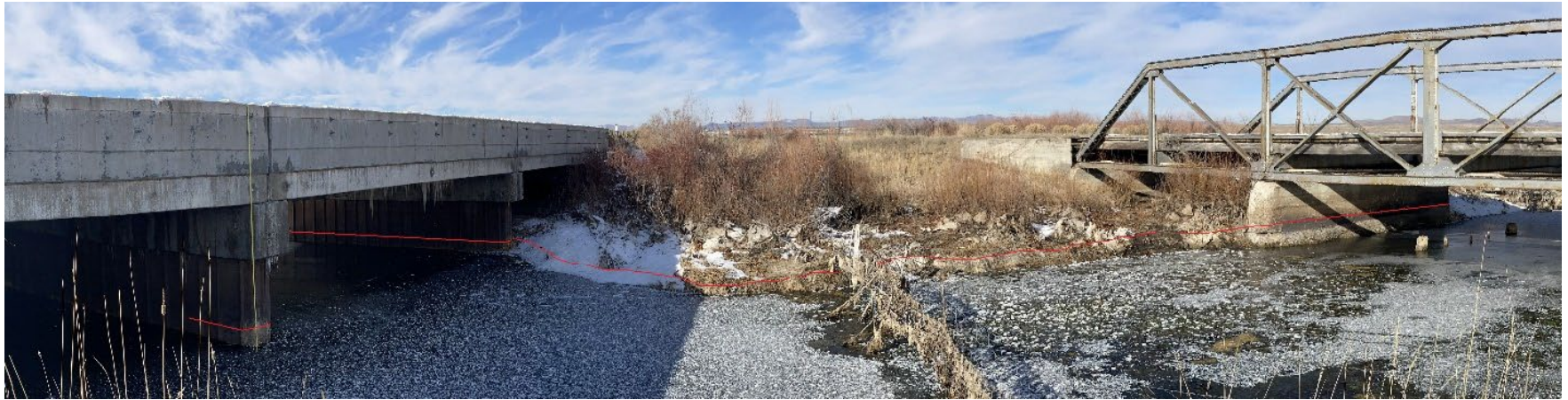
EL 1.35 B-3340 (Upstream, Looking from the East shore to the West shore)
