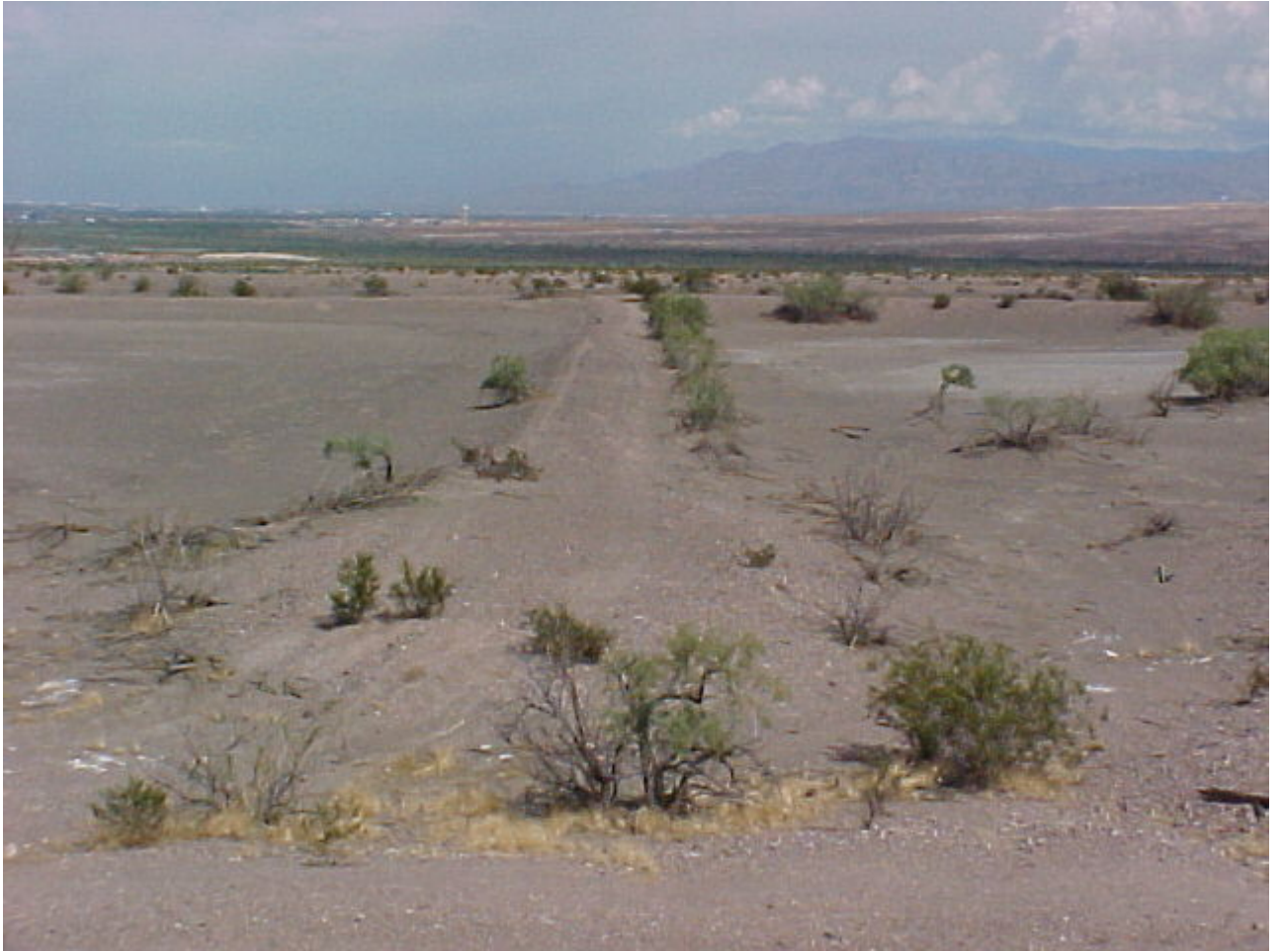
Typical berm between two ponds at the Upper Ponds portion of the Site
